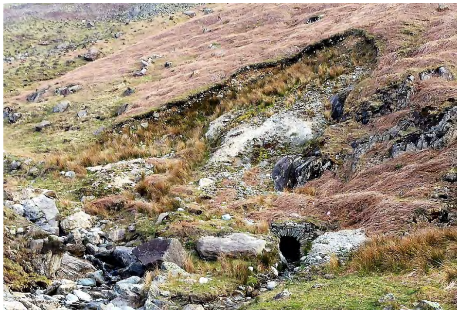
Landslip adjacent to Deep Level portal
