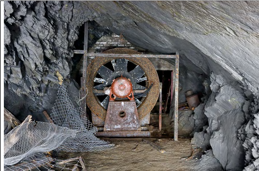
Chamber 31 ventilation fan.
