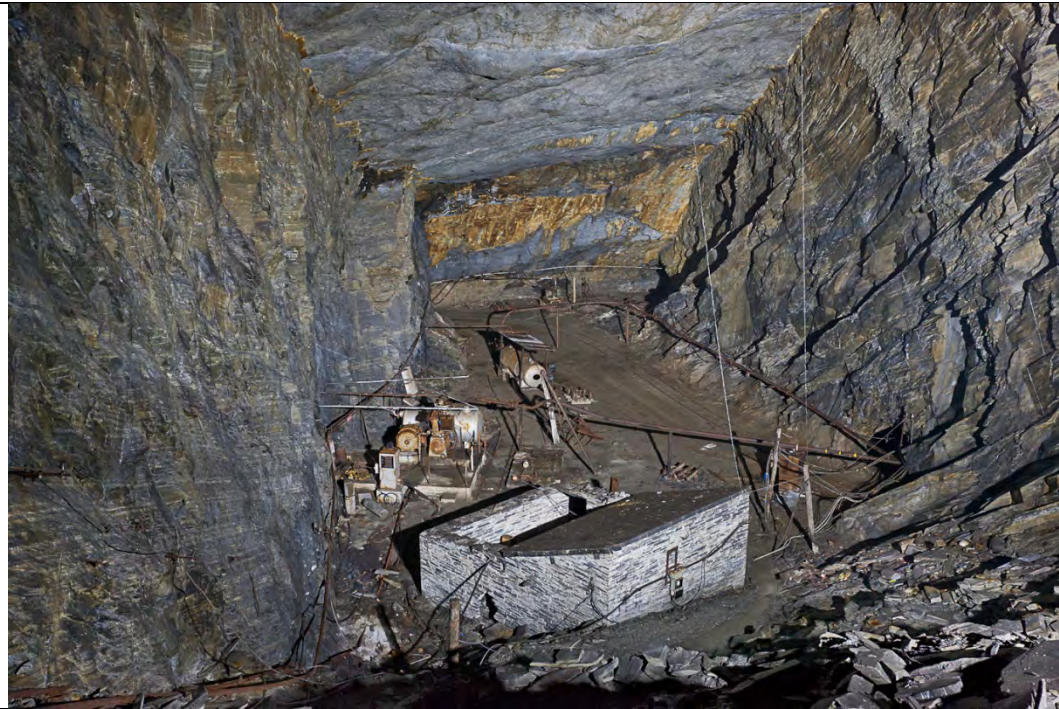
Chamber 8 Back Vein showing compressors and switchgear room.
