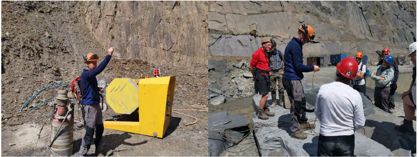
Carl shows the wire saw and how the diamond saw wire is made up with an explanation of how the holes are drilled for the wire saw to be fed through.
